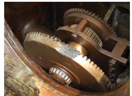
Damaged intermediate reduction gearing of the rotor turning gear
