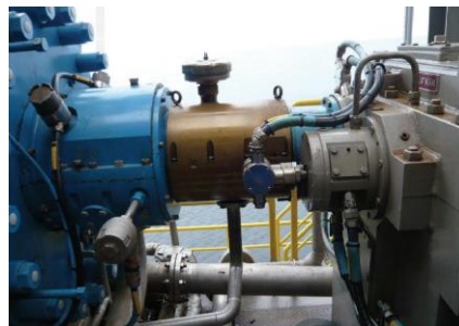
Low pressure compressor, coupling with casing and transmission of the string
